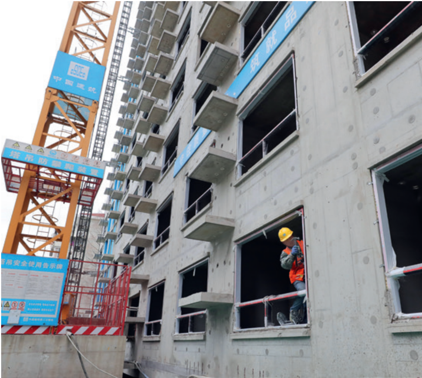
A residential complex, part of an urban renewal project, under construction in Shanghai on March 15
